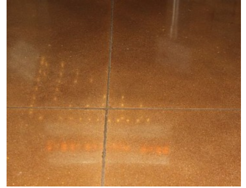
The Summit Recreation Center - Bomanite Integrally Colored Polished Concrete Floor - Close Up
