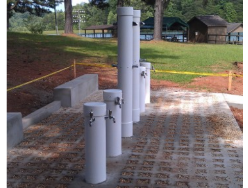
Camp Bud Schiele - Cub Scout Rinse Station - Stone Filled Grasscrete System Finished Installation
