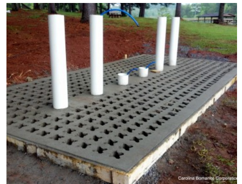
Camp Bud Schiele - Cub Scout Rinse Station - Ready for Voids to be Filled with Aggregate
