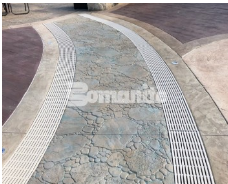
Canobie Lake Park, Castaway Island Expansion by Harrington Bomanite installation of the drainage walkway meandering brook Stamped with Bomacron Garden Stone Pattern Decorative Concrete
