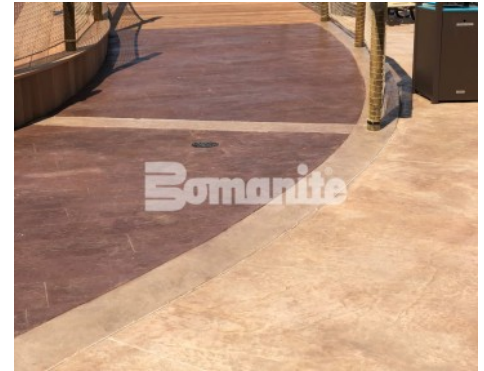
Canobie Lake Park, Castaway Island Expansion by Harrington Bomanite installation of the Tidal River Walk Stamped with Bomacron 11.5" Boardwalk Pattern Decorative Concrete
