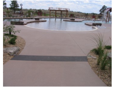
Idyllwilde Recreation Center - Mixed Use Bomanite Imprinted Concrete and Bomanite Sandstone Texture
