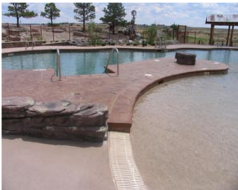
Idyllwilde Recreation Center - Mixed Use Bomanite Imprinted Concrete and Bomanite Sandstone Texture
