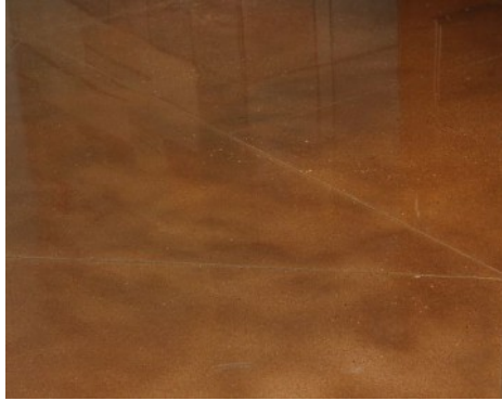
The Summit Recreation Center - Bomanite Integrally Colored Polished Concrete Floor - Close Up
