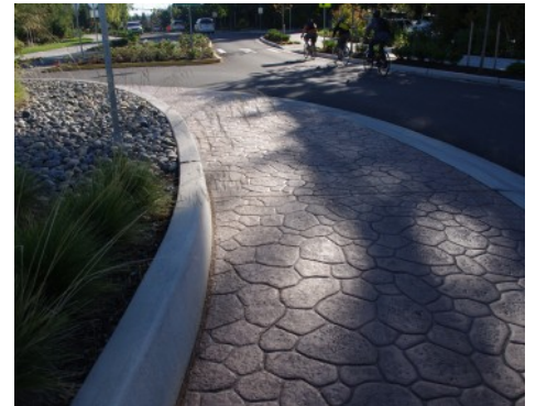
Washington NE 36th Street Bridge Roundabout - Bomanite Imprint Systems - Bomacron Creek Stone Pattern
