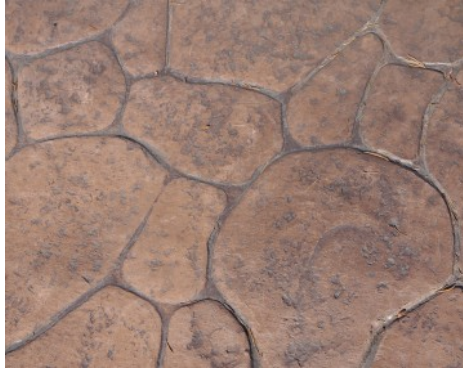
Washington NE 36th Street Bridge Roundabout - Bomanite Imprint Systems - Bomacron Creek Stone Pattern
