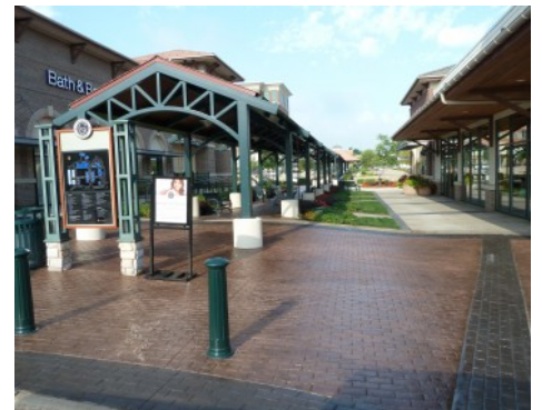
Greenway Station - Paver Replacement with Bomanite Imprint Systems
