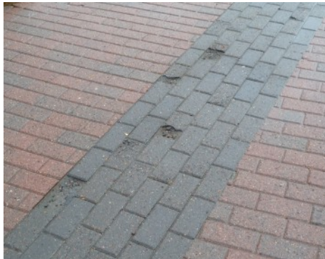
Greenway Station - Paver Replacement Before Image
