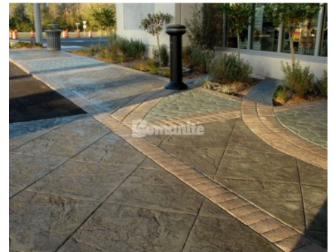
Florida Turnpike Canoe Creek - Bomanite Imprint Systems; Slate Texture, Soldier Course Brick, River Rock
