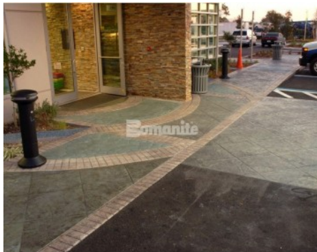
Florida Turnpike Canoe Creek - Bomanite Imprint Systems; Slate Texture, Soldier Course Brick, River Rock
