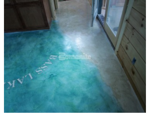
Private Residence Bass Lake - Bomanite Toppings Systems Micro-Top Base with Bomanite Con-Color
