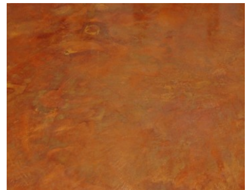
Bomanite Toppings Systems - Micro-Top with Patene Arectura Chemical Stain Interior Office Floor
