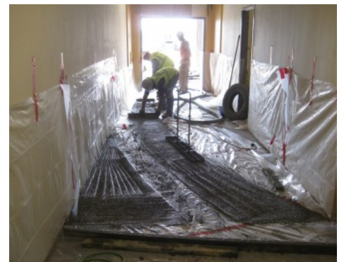
Wyoming Combined Labs - During Installation, Space Constraints
