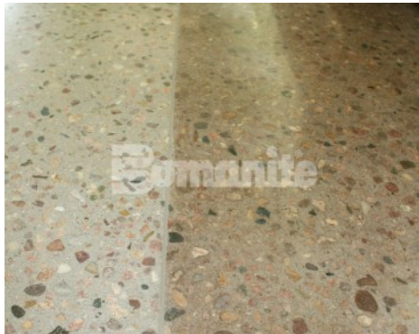
Army National Guard Windsor Colorado - Bomanite Patène Teres Polished Concrete Interior Floor
