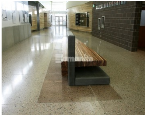
Army National Guard Windsor Colorado - Bomanite Patène Teres Polished Concrete Interior Floor
