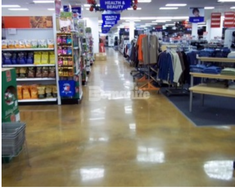
Fort Hamilton New York PX - Interior Floor with the Bomanite Custom Polishing Patene Teres System with Concrete Dye
