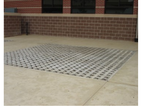
Wooster Elementary School - Exterior Walkway with a combination of Grasscrete and Imprinted Concrete
