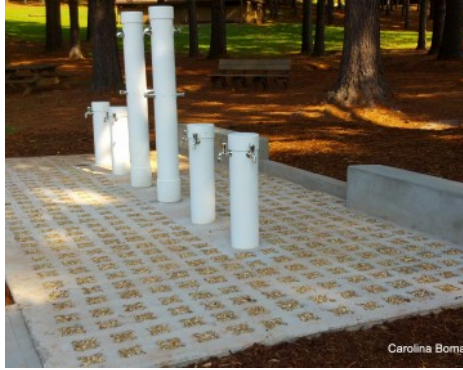
Camp Bud Schiele - Cub Scout Rinse Station - Stone Filled Grasscrete System Finished Installation
