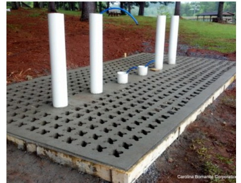
Camp Bud Schiele - Cub Scout Rinse Station - Ready for Voids to be Filled with Aggregate
