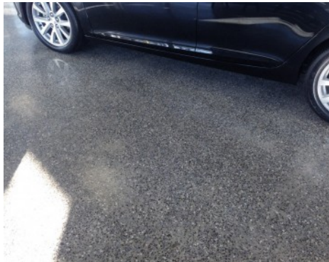
Modena by Bomanite Polished Concrete - Partyka Car Dealership using Modena Monolithic System
