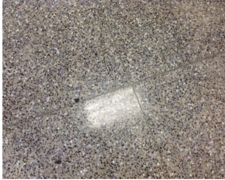
Modena by Bomanite Polished Concrete - Partyka Car Dealership using Modena Monolithic System
