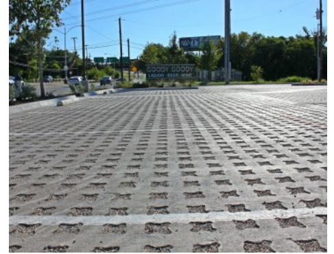
Goody Goody Liquor Store Parking Lot - Bomanite Pervious Grasscrete Stone Filled System - ADA Access
