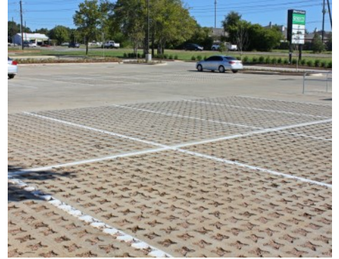
Sprouts Farmers Market Denton Tx - Bomanite Pervious Concrete Grasscrete Stone Filled System
