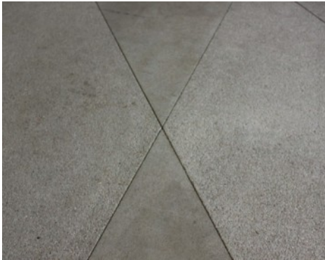
South Congress Hotel - Bomanite Exposed Aggregate Sandscape Texture and Sandblast Finishes with concrete planter walls and water features
