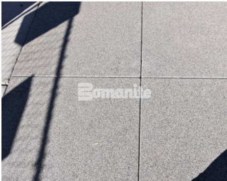
DELO - Downtown East Louisville: Exposed Aggregate Sandscape Texture Streetscape; Sandscape Refined Seat Walls
