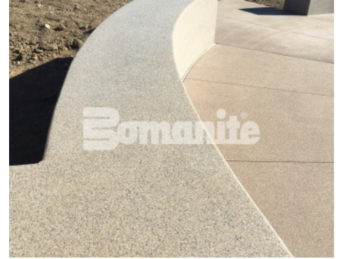
DELO - Downtown East Louisville: Exposed Aggregate Sandscape Texture Streetscape; Sandscape Refined Seat Walls
