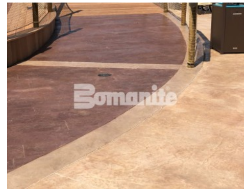
Canobie Lake Park, Castaway Island Expansion by Harrington Bomanite installation of the Tidal River Walk Stamped with Bomanite 11.5" Boardwalk Pattern Decorative Concrete
