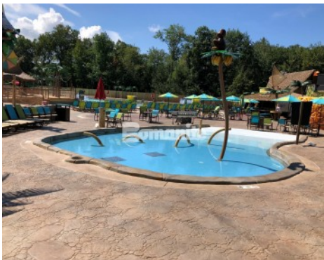
Canobie Lake Park, Castaway Island Expansion by Harrington Bomanite installation of the Kids lagoon Stamped with Bomanite Garden Stone Pattern Decorative Concrete
