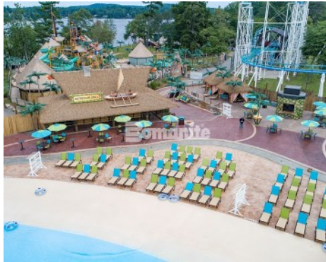
Canobie Lake Park, Castaway Island Expansion by Harrington Bomanite installation of the Walkway and Plaza Stamped with Bomanite 11.5" Boardwalk Pattern and Regular Slate Textured Decorative Concrete
