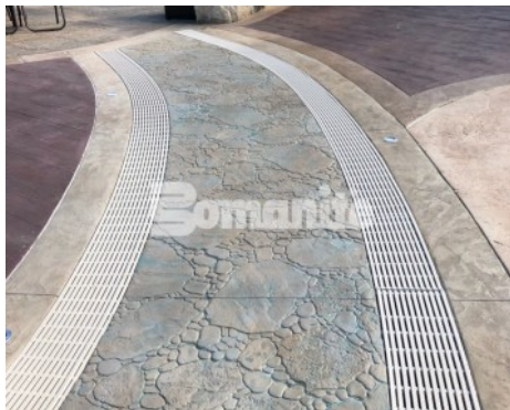
Canobie Lake Park, Castaway Island Expansion by Harrington Bomanite installation of the drainage walkway meandering brook Stamped with Bomanite Garden Stone Pattern Decorative Concrete
