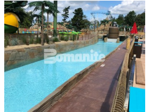
Canobie Lake Park, Castaway Island Expansion by Harrington Bomanite installation of the Tidal River Lifeguard Walk Stamped with Bomanite 11.5" Boardwalk Pattern Decorative Concrete
