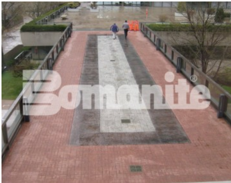
Tower Plaza - Bomanite Imprint Systems; Bomanite Basketweave Brick (no Texture) and Bomacron Medium Ashlar Slate
