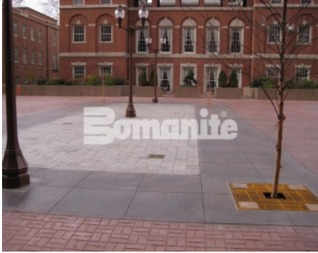
Tower Plaza - Bomanite Imprint Systems; Bomanite Basketweave Brick (no Texture) and Bomacron Medium Ashlar Slate
