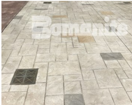
Tower Plaza - Bomanite Imprint Systems; Bomanite Basketweave Brick (no Texture) and Bomacron Medium Ashlar Slate
