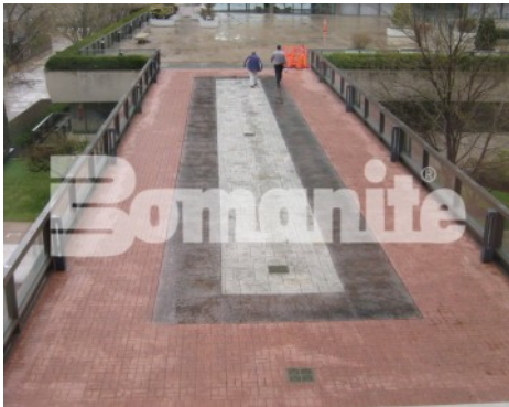
Tower Plaza - Bomanite Imprint Systems; Bomanite Basketweave Brick (no Texture) and Bomacron Medium Ashlar Slate
