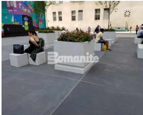
World Trade Center New York Tower 2 Street Design - Bomanite Alloy Exposed Aggregate System
