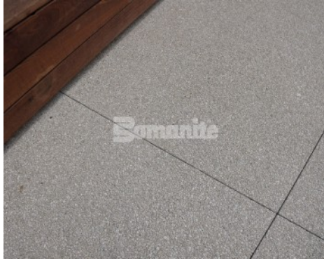
Flight at Tustin Legacy Business Development Campus - Bomanite Exposed Aggregate Revealed Walkway Close Up
