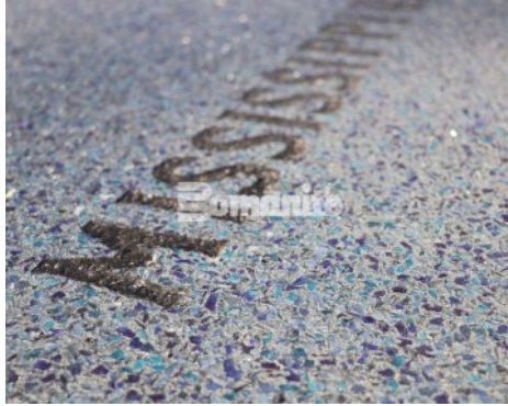
St. Louis Aquarium at Union Station - Bomanite Revealed Exposed Aggregate River Confluence Entry
