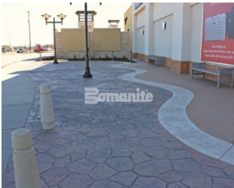
Target Outlets Fort Worth - Bomanite Imprint Systems Walkways - Canyon Stone, Used Brick Texture, Broom Finish
