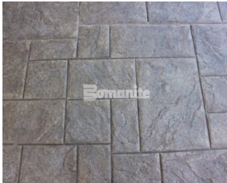
Target Outlets Fort Worth - Bomanite Imprint Systems Walkways - Medium Ashlar Slate Pattern
