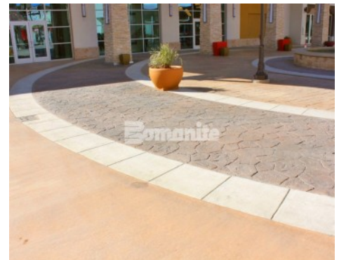
Target Outlets Fort Worth - Bomanite Imprint Systems Walkways - Canyon Stone, Used Brick Texture, Broom Finish
