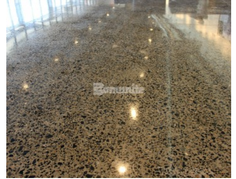
Chase Oaks Church Fairview TX - Bomanite VitraFlor Polished Concrete with Black Aggregates
