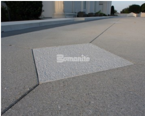
Church of Jesus Christ of Latter Day Saints in Windermere, FL, Exposed Aggregate installed by Edwards Concrete Bomanite.
