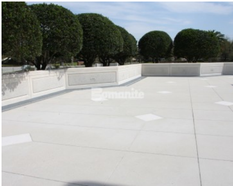
Church of Jesus Christ of Latter Day Saints in Windermere, FL, Exposed Aggregate installed by Edwards Concrete Bomanite.
