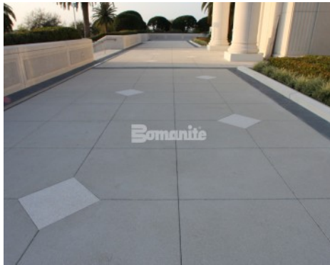
Church of Jesus Christ of Latter Day Saints in Windermere, FL, Exposed Aggregate installed by Edwards Concrete Bomanite.
