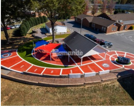
Statesville Christian School in NC featuring Micro-Top XT installed by Carolina Bomanite Corporation.
